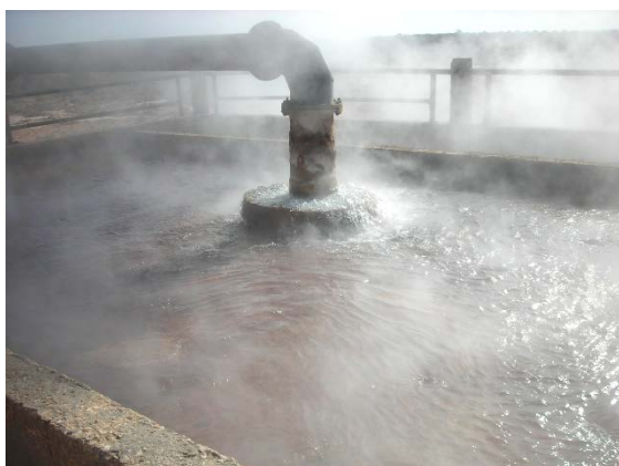
Fig.3 : Water outlet on the cooler.
